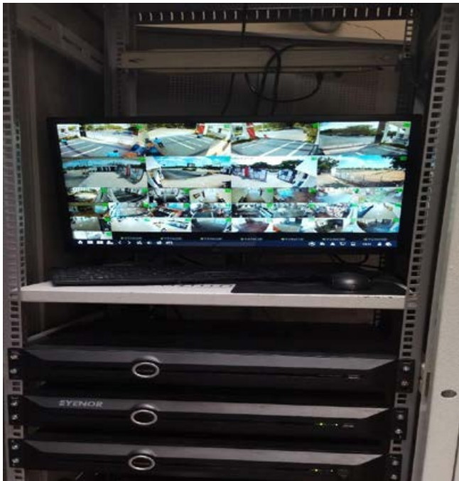
CCTV Feeds Network Video Recorders
